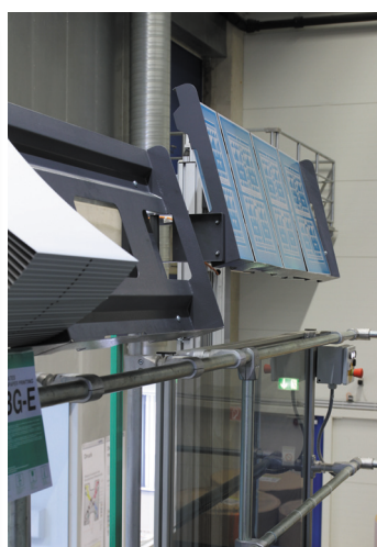
At the press gallery, plates are stored on a plate rack, awaiting the next plate change.
